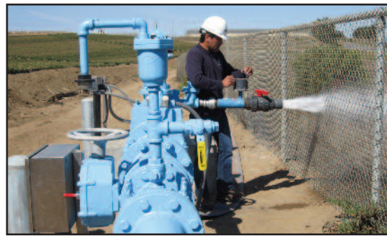
Senior Water System Operator, Jesus Martinez, tests the new Harkin's Slough well and appurtenances*
